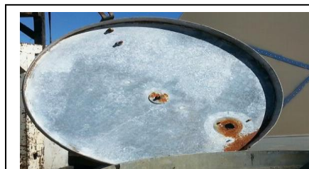
An example of the “vent” cut into the man-way cover of a light gage welded tank. Notice the corrosion around the vent hole where the galvanization was burned off.
